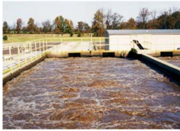
Figure 20.46: Aeration tank showing the activated sludge process. © 2004 Pearson Education, Inc.
